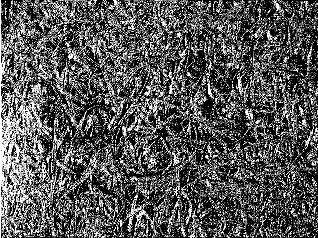
Southaven, fiberboard ceiling detail, 4421Richard Circle, July 24, 2012 (Photograph by Charles J. Fisher)
