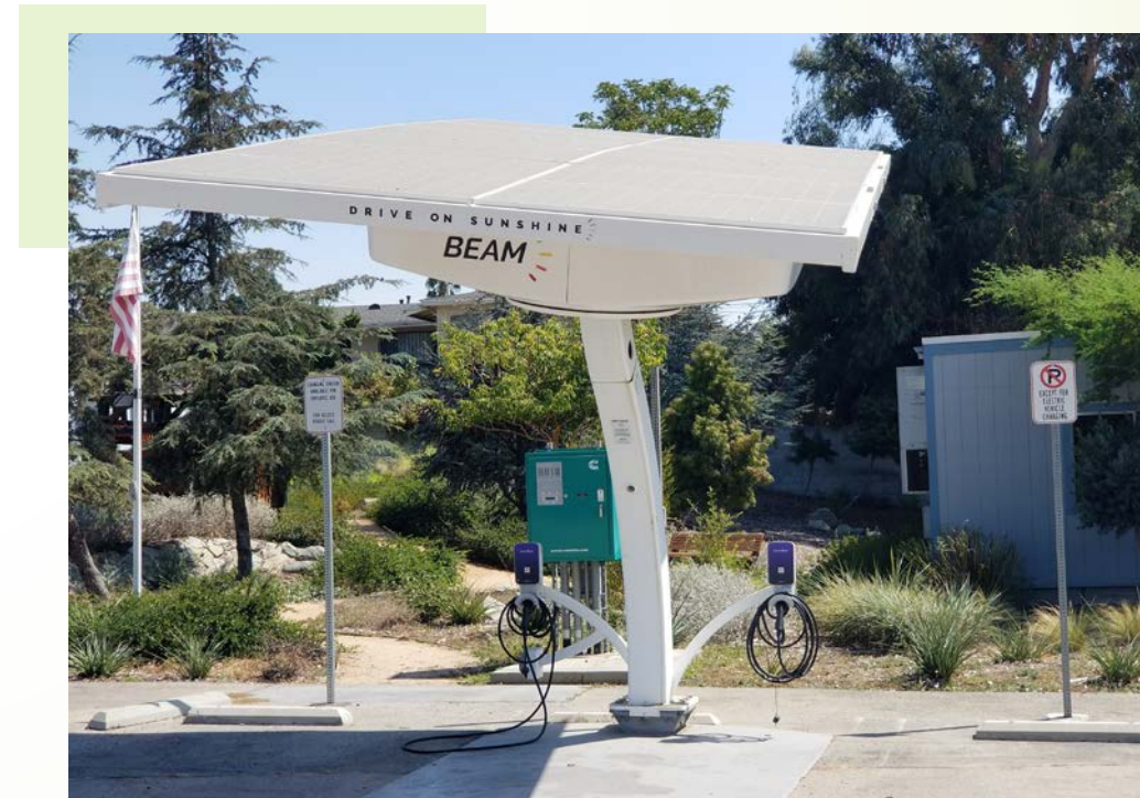
Solar powered charging station
